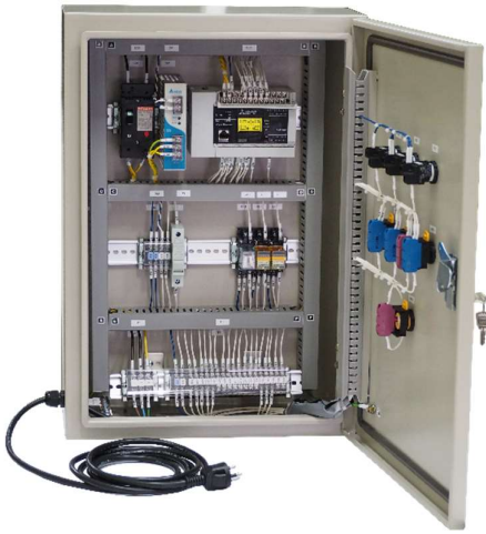
Control Panel (MC-01)
